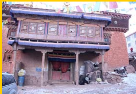
Above: the existing main temple where the nuns gather to perform 20 drubchens * a year. Currently, the structure is at risk of collapsing. This year the construction for a new temple will begin!
